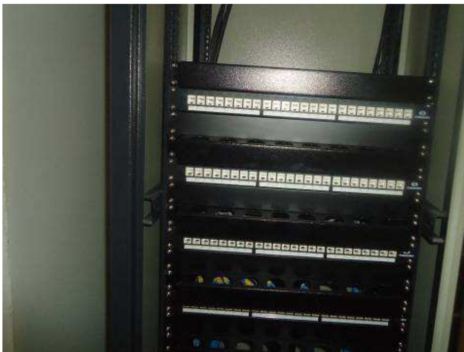
RACK, PATCH PANEL DATA: AGOSTO/2017
